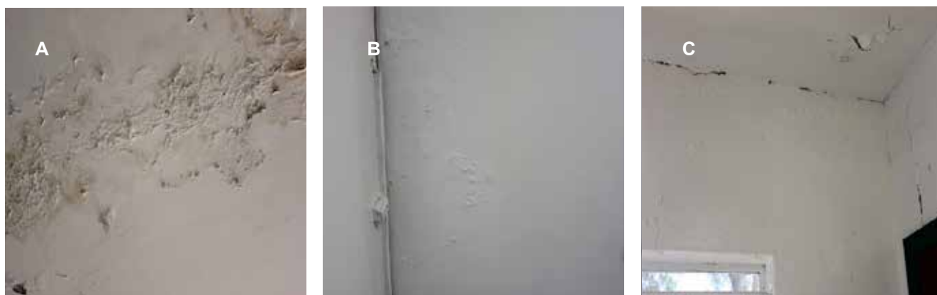
Figure 2: Water-damaged walls and ceilings observed during an inspection in some of the work areas of the patient: (a) tearoom, (b) patient's office, and (c) laboratory.
